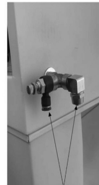
Push Lock fitting and elbow pointing downward
