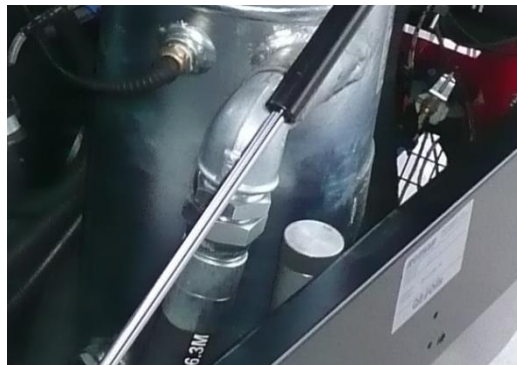
Figure 10.1-1 Checking the oil level in the compressor
