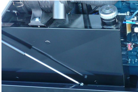
Figure 10.1-2 Fuel tank for Diesel engine
