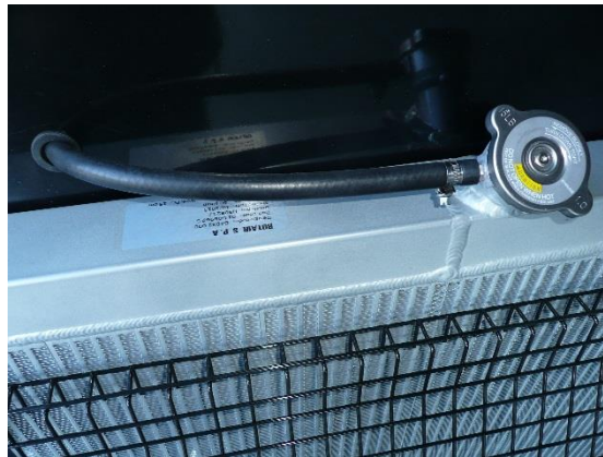
Figure 10.1-3 Checking the radiator cooling liquid
